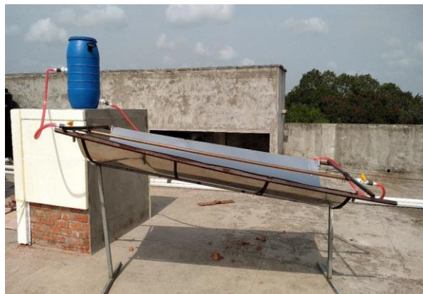
Fig.4 The solar collector setup.
